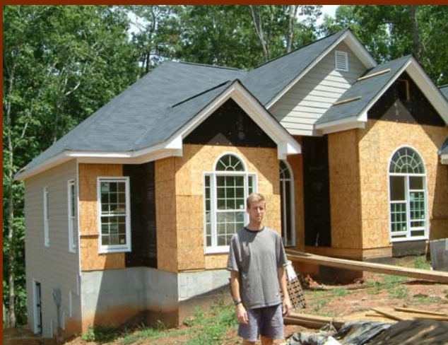
Jim Casey in front of the radon resistant house he is building in Athens.
