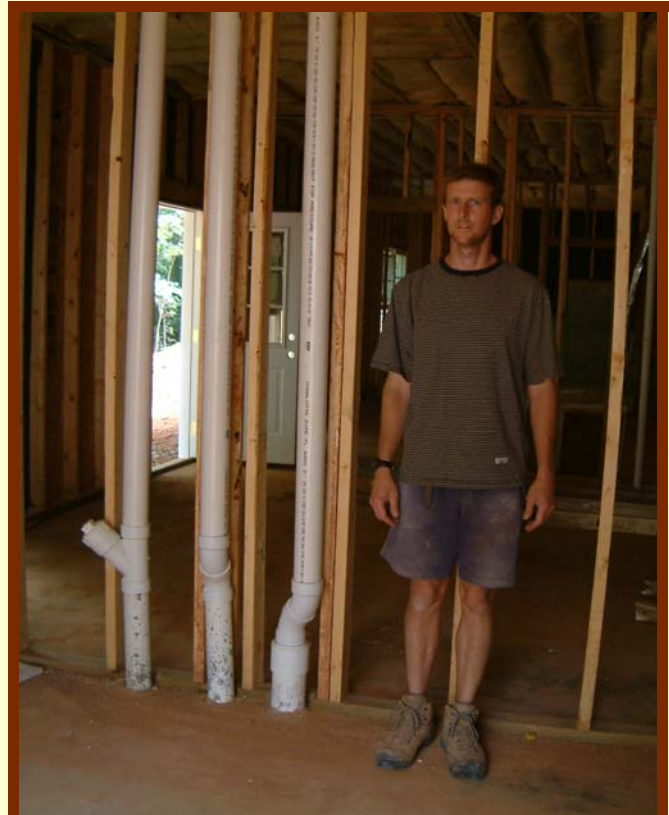
Jim Casey standing by the radon vent stack (the radon pipe is the one on the right) in the basement of the new house.
