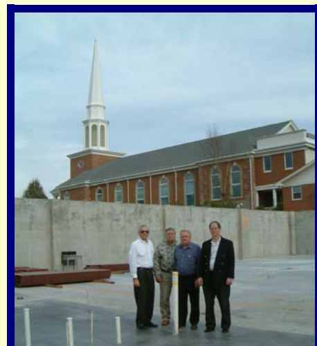
The Mars Hill Church multi-purpose building will have radon vent stacks to divert radon gas from under the foundation to the outside air where it will be diluted.
