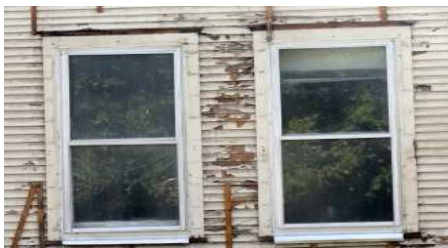
Peeling Lead Paint. Image Source: Pamela Turner
